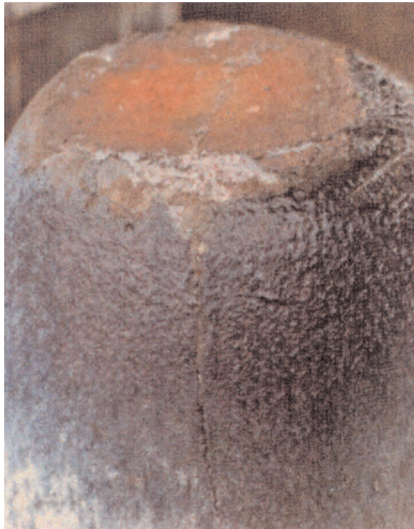
Crack caused by the incorrect use of parting agents.
