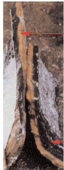
Layer of oxidation.
